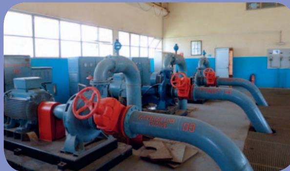
Station de pompage hydraulique, Dakar © AFD – Hélène Cure
